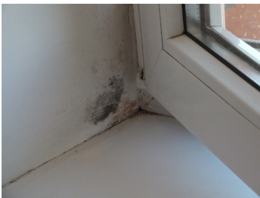
Figure 10. Humidity condensation and mold formation on the internal surface of the coupling joint between window and the wall opening
