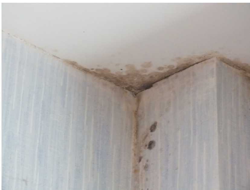
Figure 9. Humidity condensation and mold formation on the internal surface of the coupling joint between the column and the inter-floor slab
