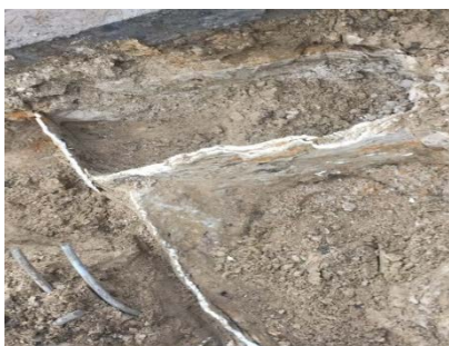
Figure 15. A section of the injected plot after the injection of the resin (The investigated soil and the resin propagation)
