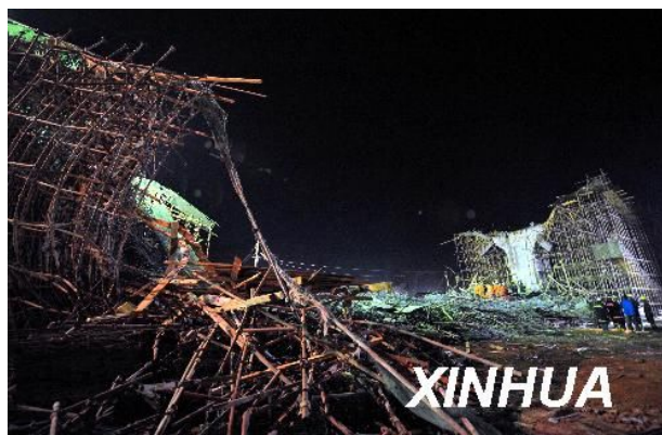
Figure 1. Collapse of FSTFHS system during construction in Yunnan Province on January 3, 2010.
