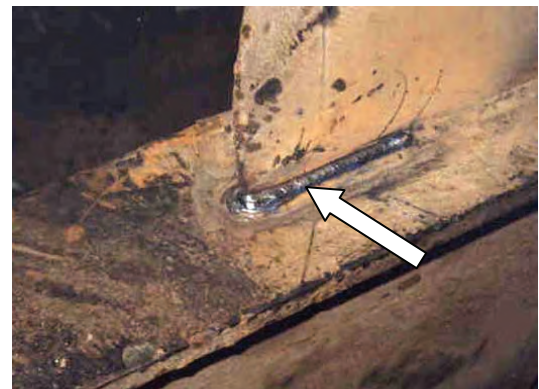
Fig. 1. Fatigue crack (re-welded) at the bracket ending on the flange of longitudinal stiffener. A tanker ship bottom structure. Courtesy of Lloyd's Register
