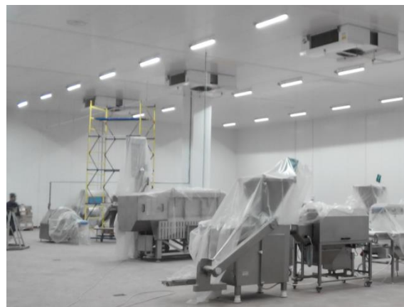
Figure 8. Installed air-cooling devices
