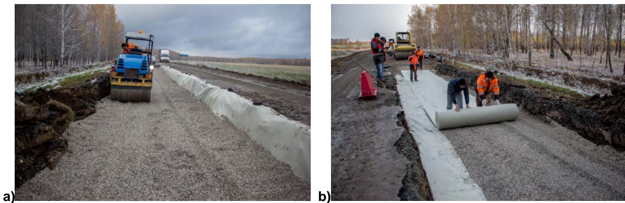
Figure 6. Construction of the experimental section with GC: a – GC compaction by roller; b – geotextile laying above GC
