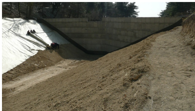
Figure 23. A view of the above-ground reservoir from the upstream side while performing the works of waterproofing
