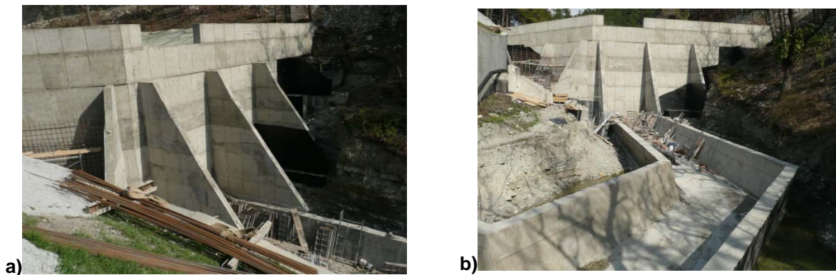
Figure 22. View of the above-ground reservoir from the downstream side at completion of construction
