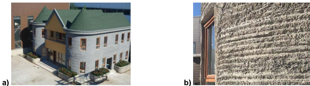
Figure 3. Typical 3D printing defects on the example of residential building by 'Tengda' (China) [12]: a), b) disruption of the geometrical dimensions due to spreading of the underlying layers, surface heterogeneity.
