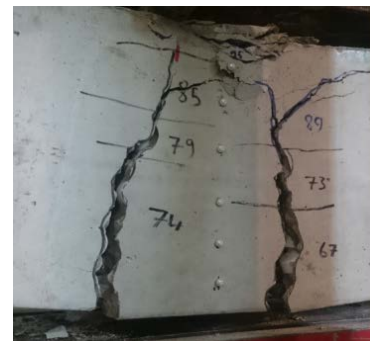
Figure 12. Flexural cracks for 10 % PBC beam.
