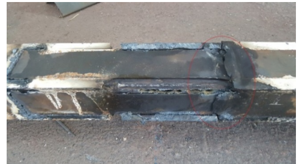
(b) tearing of brace at the end of the fuse
