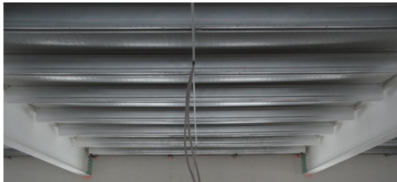
Figure 2. Bottom view of the floor slab of the second floor: significant deflections of the ribs of the profiled steel sheet.
