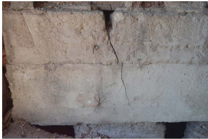
Figure 2. Cracks in the foundation.
