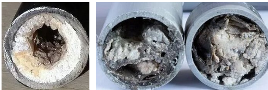
Figure 1. Partially or completely clogged sewer pipes [4–8].
