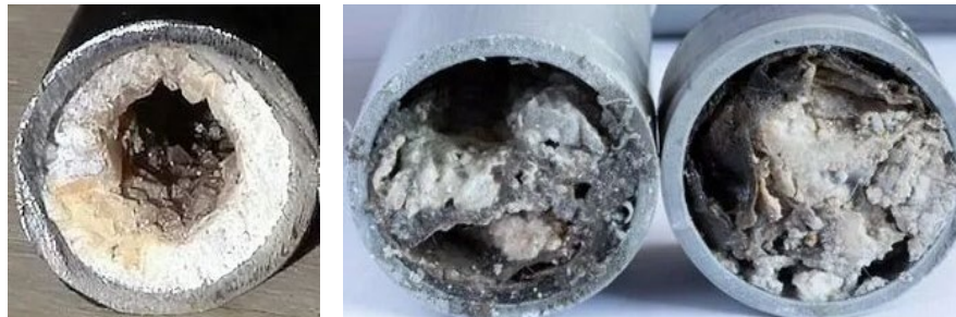
Figure 1. Partially or completely clogged sewer pipes [4–8].
